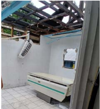
Fire damage to a radiology room
